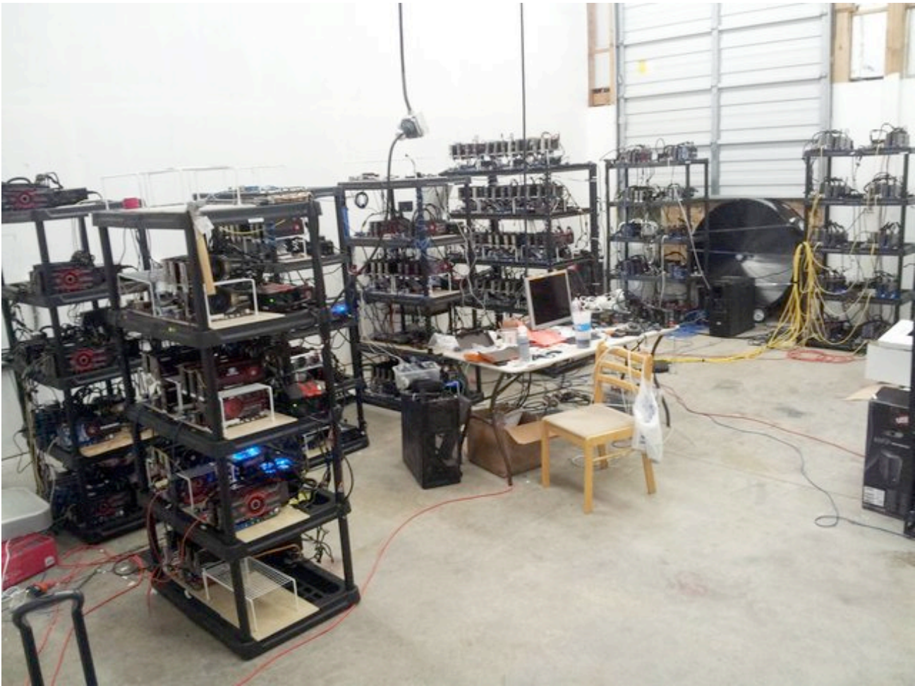
Figure 3. Photograph of a Bitcoin mining server farm.
